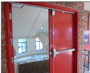
Photo of fire safety equipment Fire door.JPG
