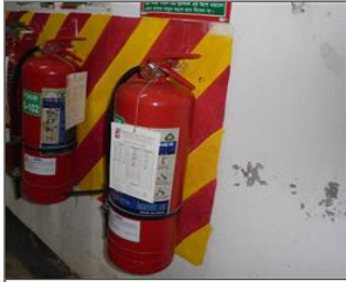
Photo of fire safety equipment Fire extinguisher.JPG
