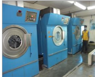
Photo of the inside of the main production hall Drier section.JPG
