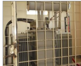
Photo of the inside of the main production hall Transformer.JPG
