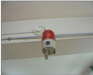
Photo of fire safety equipment Visual fire alarm.JPG
