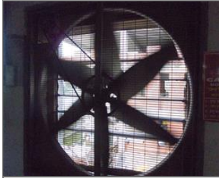
Photo of fire safety equipment Exhaust fan.JPG
