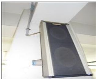
Photo of fire safety equipment PA System.JPG
