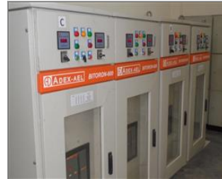
Photo of the inside of the main production hall Substation.JPG
