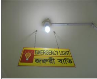
Photo of fire safety equipment Emergency light.JPG
