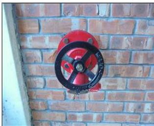
Photo of fire safety equipment Hydrant point.JPG
