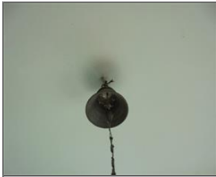
Photo of fire safety equipment Gong bell.JPG
