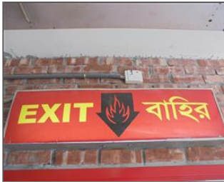
Photo of fire safety equipment Exit sign.JPG
