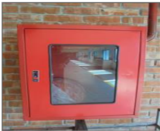
Photo of fire safety equipment Hoose reel .JPG
