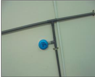
Photo of fire safety equipment Smoke detector.JPG
