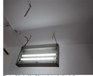
Photo of the inside of the main production hall Pest control system.JPG
