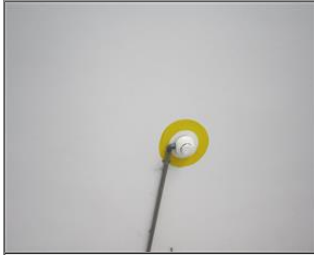
Photo of fire safety equipment Smoke detector.JPG
