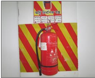
Photo of fire safety equipment Fire extinguisher.JPG
