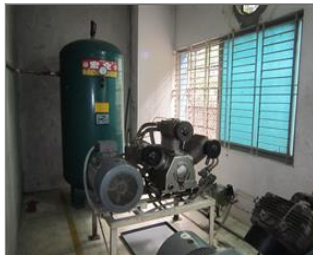
Photo of the inside of the main production hall Compressor.JPG
