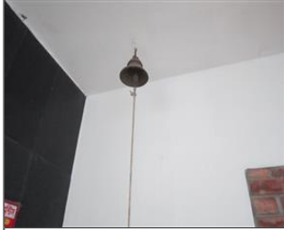
Photo of fire safety equipment Gong bell.JPG
